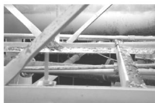
Figure 34. Dust accumulation on roof trusses.
