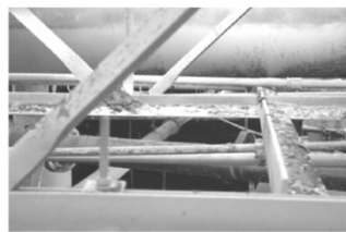
Figure 34. Dust accumulation on roof trusses.
