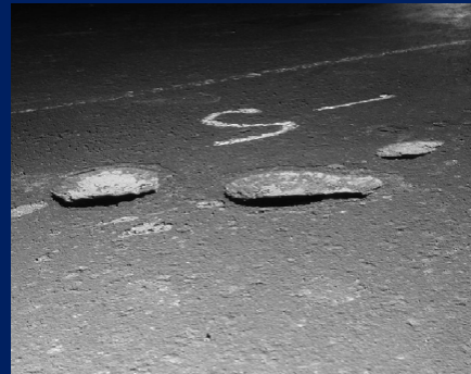
Microbiologically Influenced Corrosion
