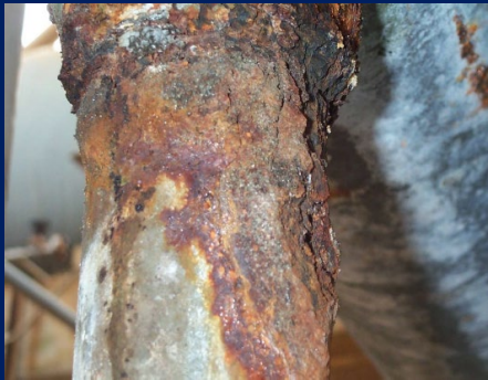
Corrosion Under Insulation
