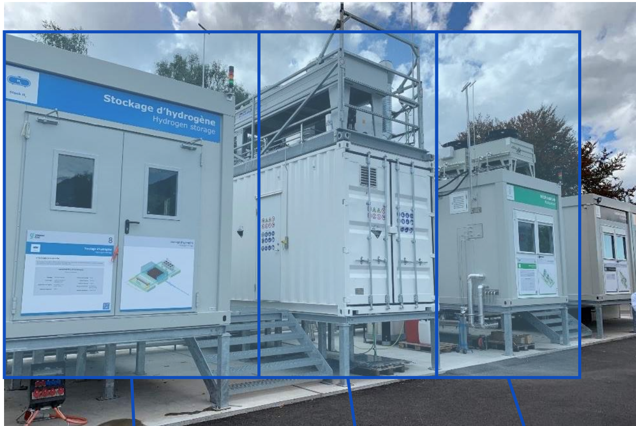
Hydrogen buffer storage (DASH technology)
