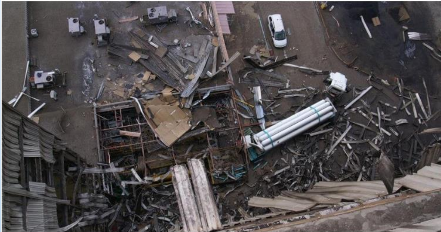
Muskingum River Power Plant explosion
