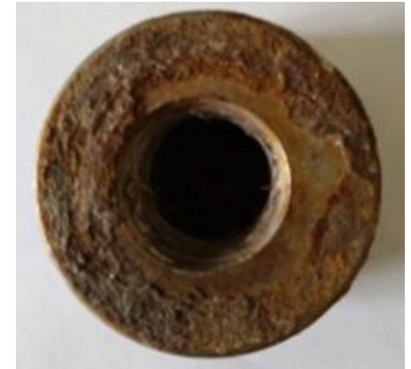
Stray current corrosion of bottom part of a bush made of super-duplex
