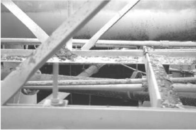
Figure 34. Dust accumulation on roof trusses.
